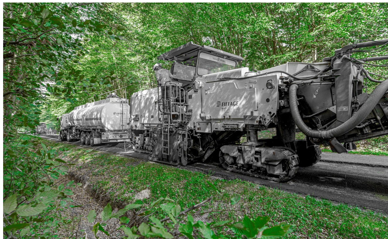
Renovation works for the D96 departmental road (Seine-et-Marne), including full recycling of road surfaces in situ, and the use of the Recytaal® certified bio-sourced binder.
