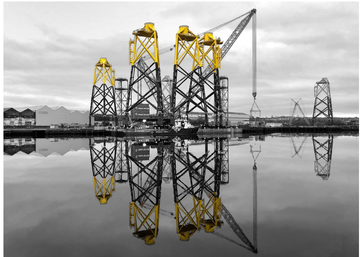
Smulders construction site in Hoboken (Belgium) View of the wind turbine foundations for the Moray East offshore wind farm (Scotland)
